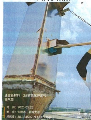
〇1 2#软氮化炉废气 DA002 排气筒
