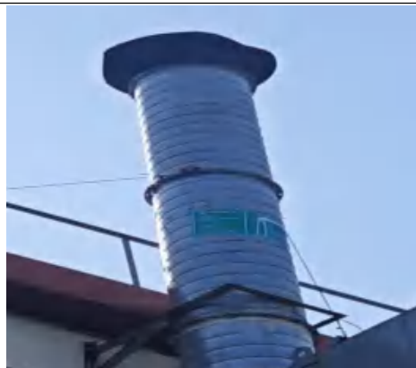
废气排放口标识标牌
